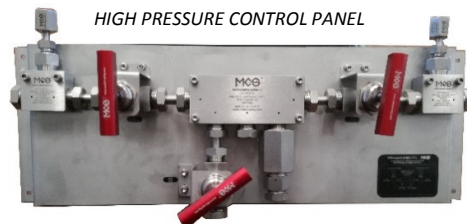
HIGH PRESSURE CONTROL PANEL
